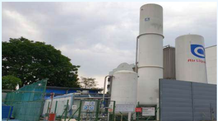
Process Nitrogen Plant
