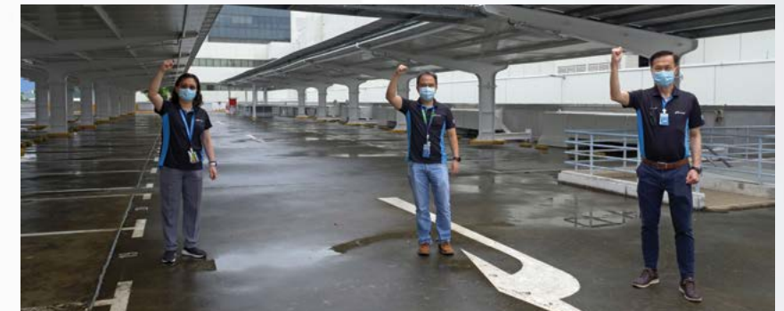
Solar panels on the Woodlands carpark, admin building, and CUP building rooftop at the Micron Singapore site were turned on in July 2021.
