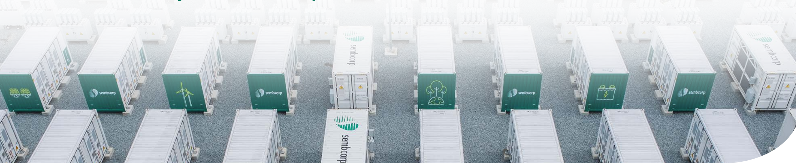
Sembcorp Energy Storage System on Jurong Island
