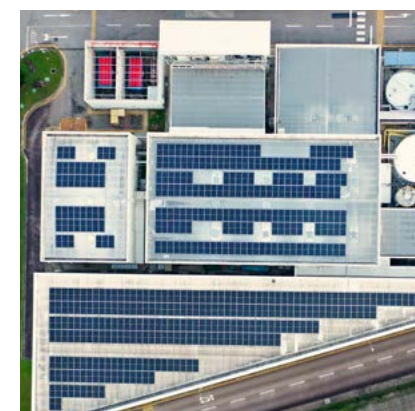
Sembcorp's rooftop solar PV asset on top of Micron Technology's plant in Singapore
