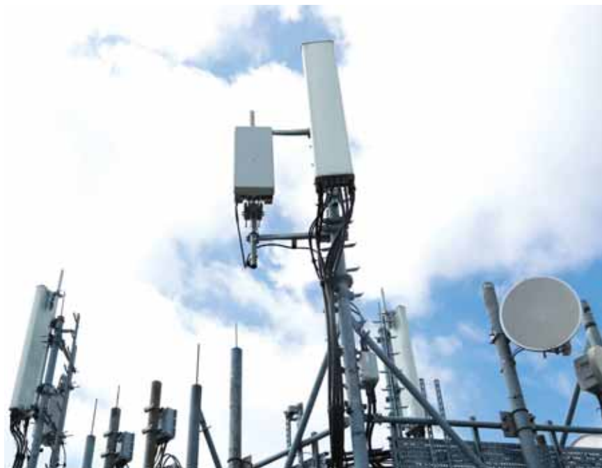
New Active Antenna Units (AAUs)
