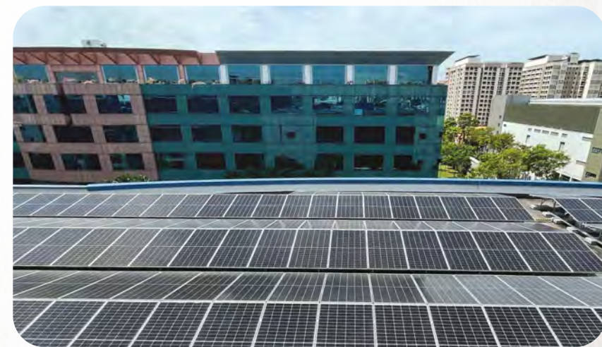
UTAC's rooftop installation will generate over one million kWh of green energy annually
