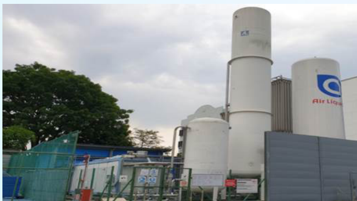
Process Nitrogen Plant
